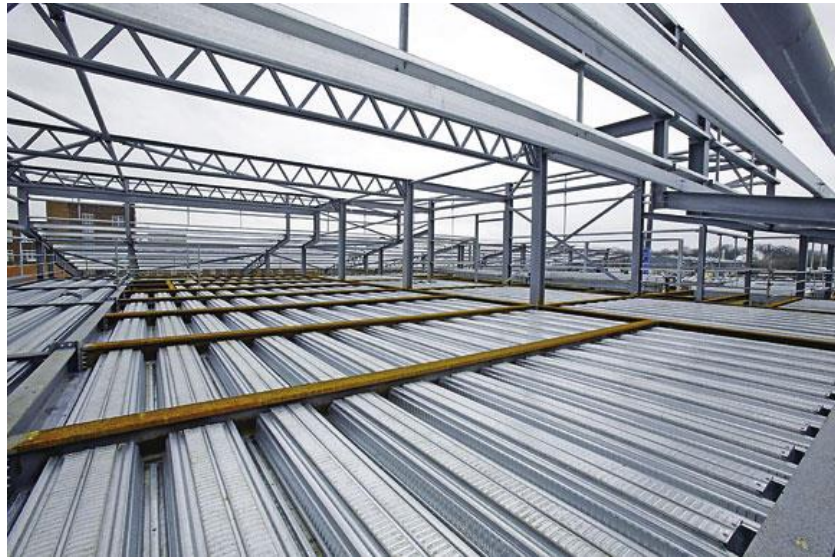
Figure 1.2. A typical example of composite slab construction, showing the deck placing on a steel frame.
