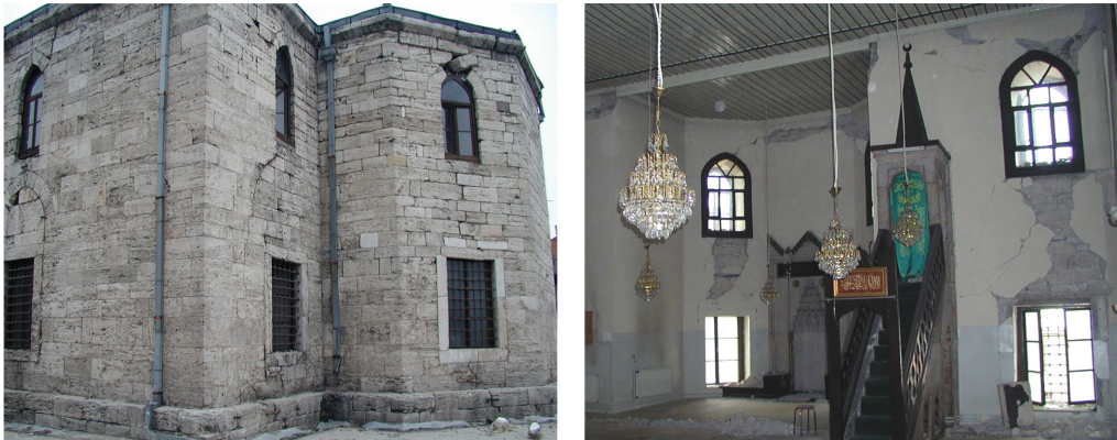
Fig. 4 Damage to southwest walls of Kadi mosque (outside and inside views)
