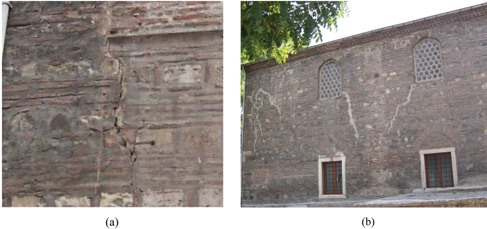
Fig. 2 (a) Vertical wall crack observed after the 1999 earthquakes and (b) repaired cracks in the Imaret mosque
