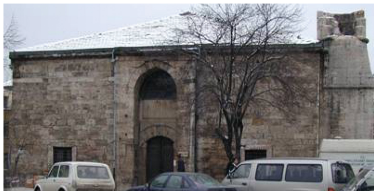
Fig. 5 Entrance of Kadi mosque showing failed minaret
