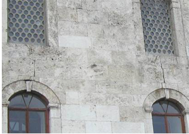
Fig. 11 Cracks in south walls of Yildirim Bayezid mosque
