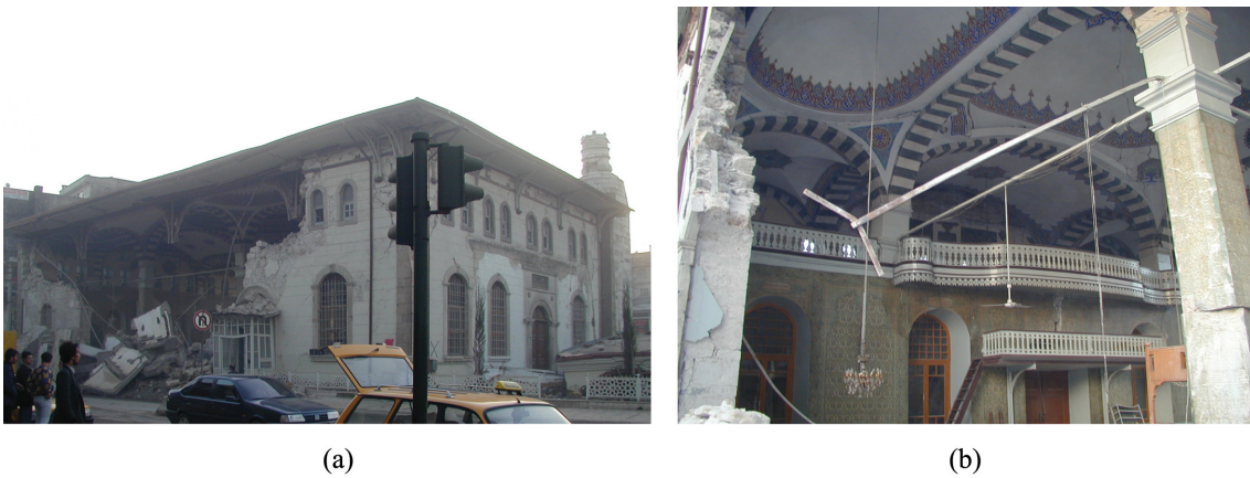
Fig. 12 Damage in the Duzce Merkez mosque after the November 12, 1999 earthquake
