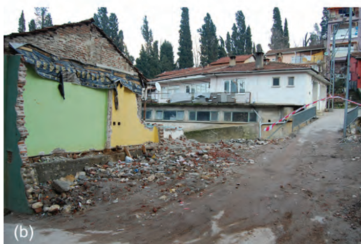
PHOTO 6A AND PHOTO 6B Demolition work in settlements where buildings are expropriated
