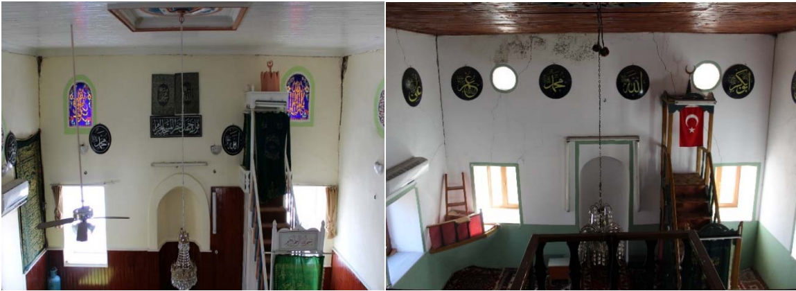
Figure 19: Observed damages at intersection of perpendicular walls
