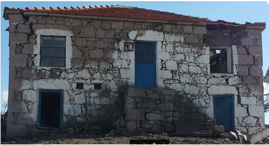
Figure 17: An example of a damaged dwelling due to inadequate interlocking
