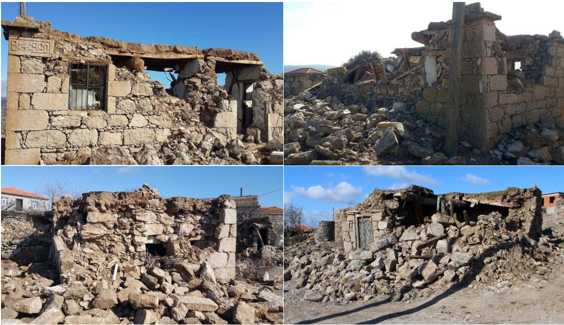
Figure 21: Examples of collapse due to heavy earth wall-roof collapse
