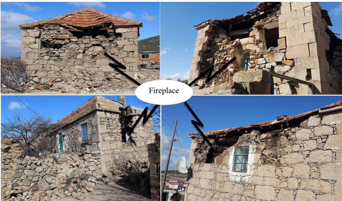
Figure 20: Examples of out of plane collapse due to wall cavity
