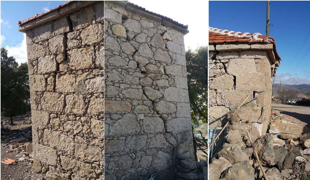
Figure 23: Examples of diagonal shear cracking
